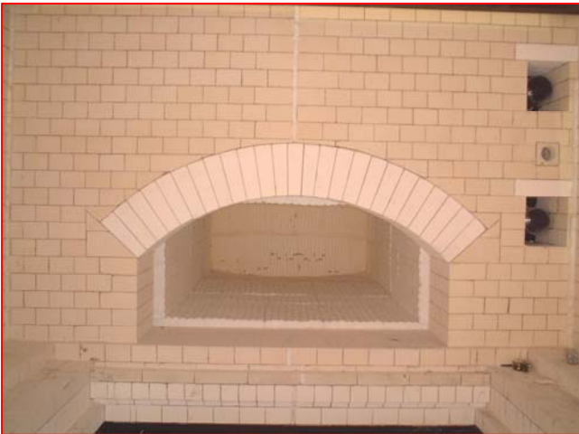
Exhaust flue to afterburner
